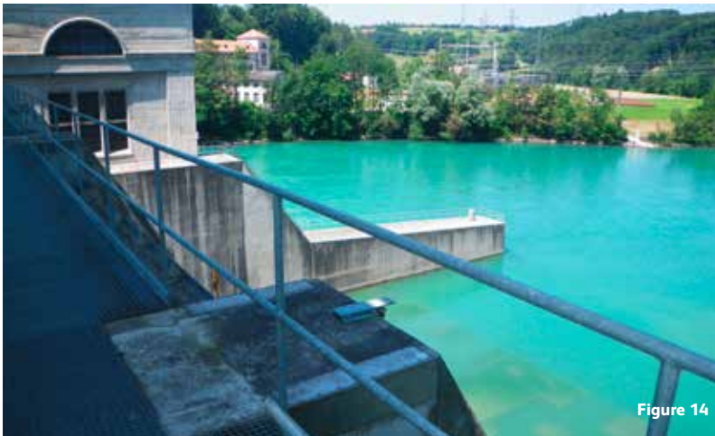
Investigation of galvanic corrosion at a run-of-river power plant
